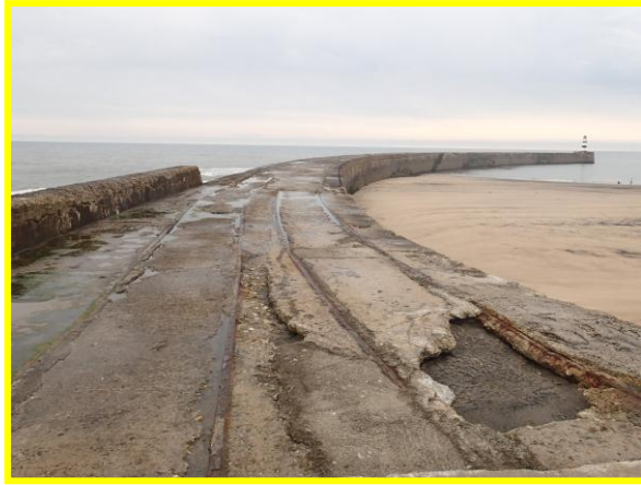
View of North Pier in 2014 showing increased damage to deck. (Asset Ref. No. 121AC901C0104C03)
