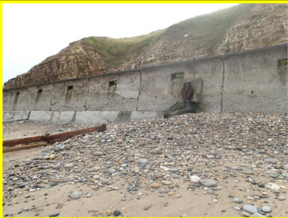
Low beach levels exposing toe of wall and damaged groynes. (Asset ref. No. 121AC901C0102C01)
