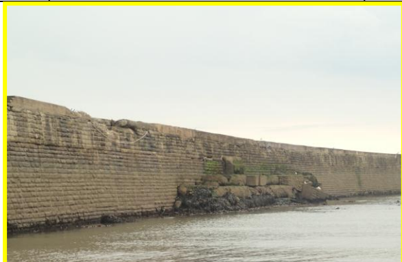
Missing section of inner coping to North Pier. (Asset Ref. No. 121AC901C0104C03)
