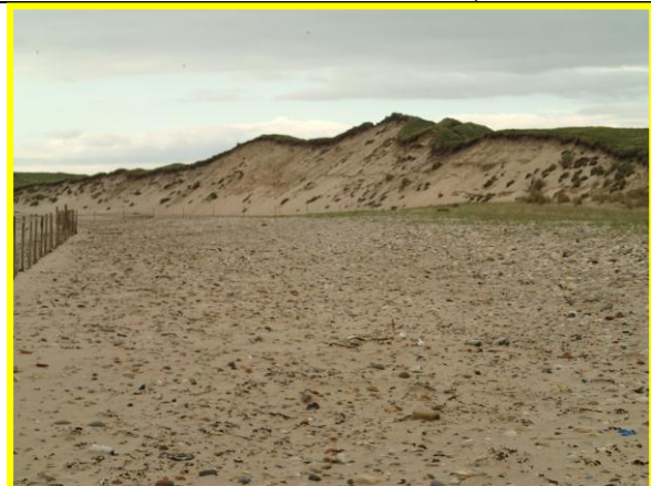
Erosion of dune face immediately south of Crimdon Beck. (Asset Ref. No. 121AC901C0301C02)
