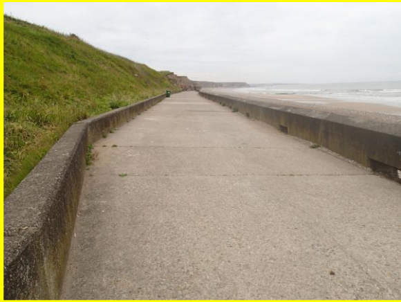
Cracks to promenade with vegetation growth. Well vegetated cliff to rear. (Asset ref. No. 121AC901C0102C01)
