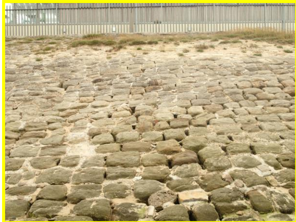
Gaps and missing grout in masonry revetment adjacent to new marina building. (Asset Ref. No. 121AC901C0104C05)
