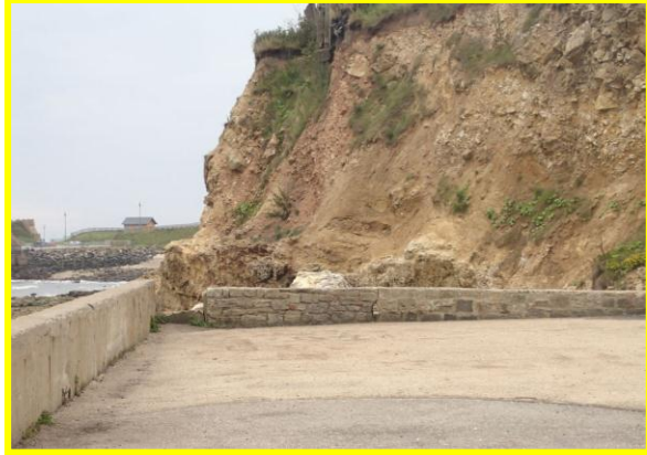
Damage to masonry at south corner of wall. (Asset Ref. No. 121AC901C0103C04)
