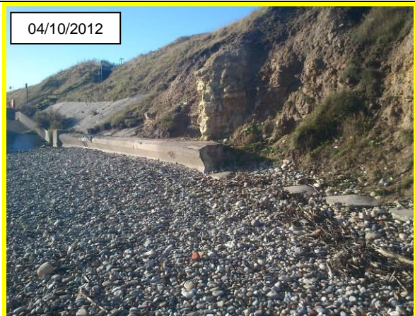
04/10/2012 Wall at north end of Seaham. Photo from 2012 report.
