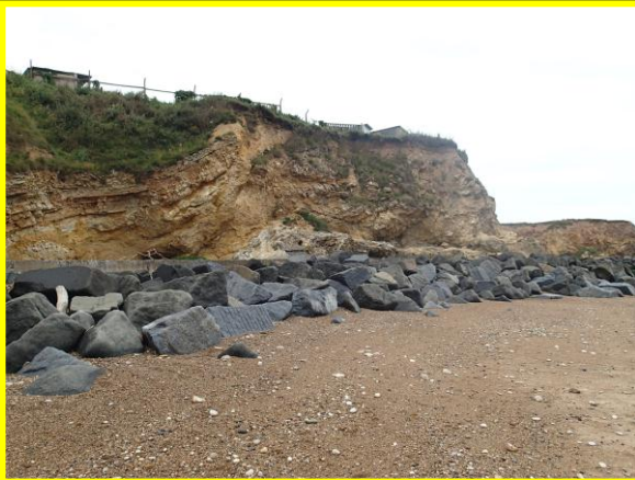
Rock armour protecting cliff toe, property sheds close to edge. (Asset Ref. No. 121AC901C0103C02)
