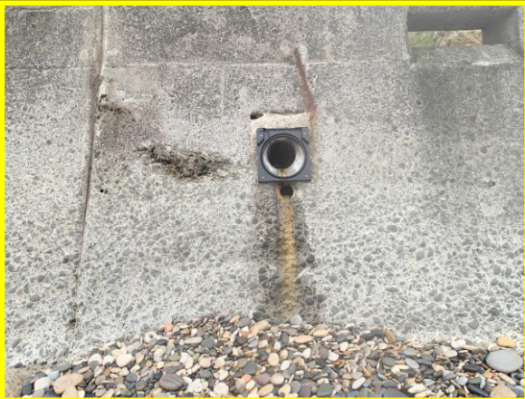
Minor abrasion damage to lower wall and example of broken flap valve. (Asset ref. No. 121AC901C0102C01)
