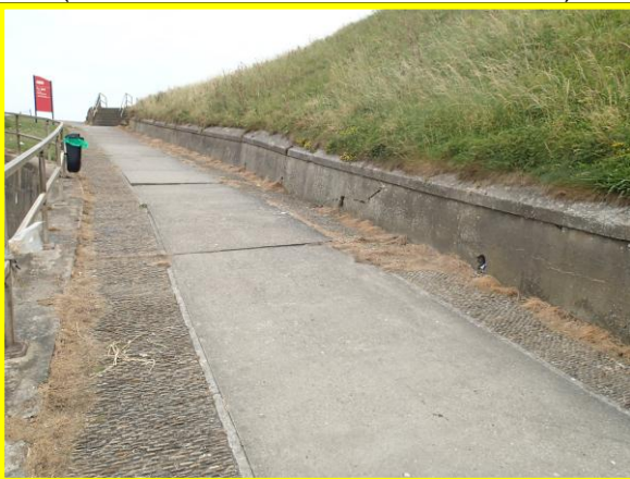
Cracking in the retaining wall to rear of beach access ramp. (Asset Ref. No. 121AC901C0103C07)
