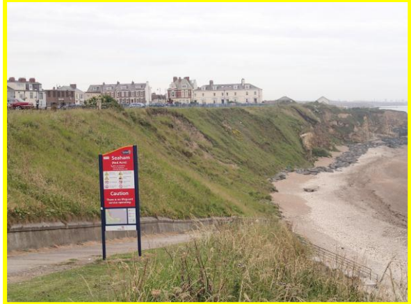
Slumping in cliff between end of rock armour and beach access steps. (Asset Ref. No. 121AC901C0103C06)
