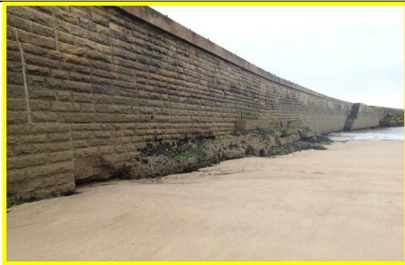
Toe erosion damage where North Pier ties into rock outcrops. (Asset Ref. No. 121AC901C0104C03)
