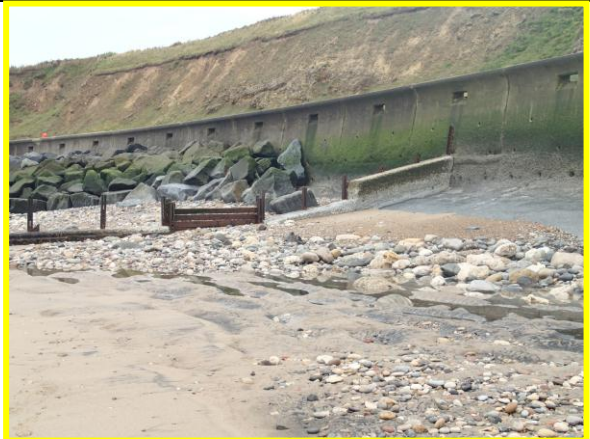
Exposed concrete toe apron adjacent to start of rock armour at south of defence. (Asset ref. No. 121AC901C0102C01)
