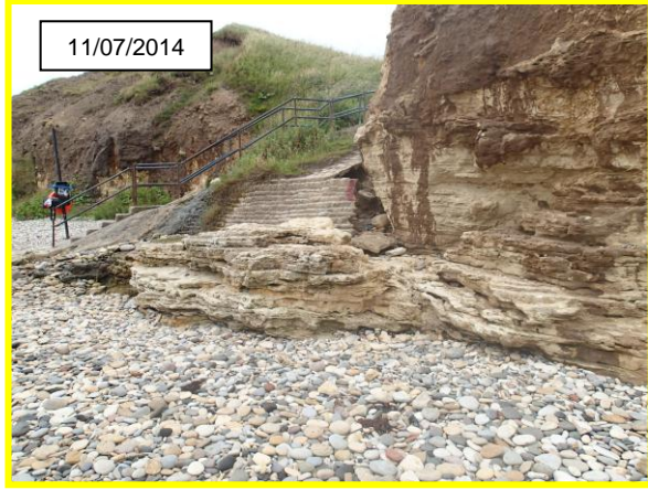
11/07/2014 Outflanking at north of steps unchanged from 2012. (Asset ref. No. 121AB901B0804C01)
