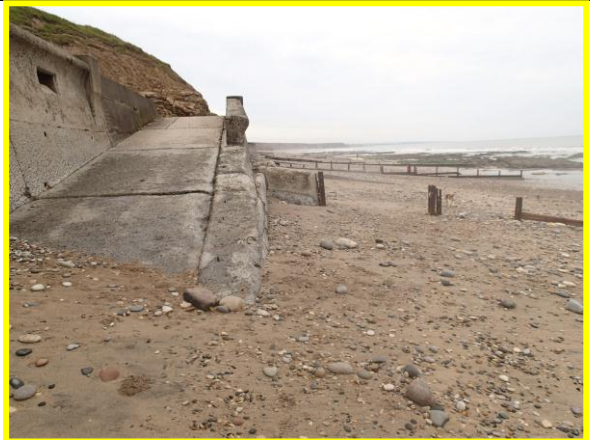
Damaged / derelict groynes on beach at south end. Recommended to confirm redundant and remove to reduce H&S risks or replace / repair. (Asset ref. No. 121AC901C0102C01)
