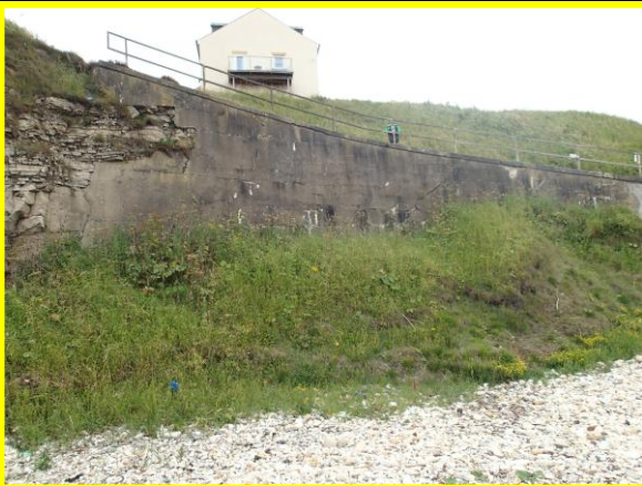
Cracking in the retaining wall to the beach access ramp. (Asset Ref. No. 121AC901C0103C07)
