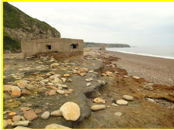
Eroding spoil beach adjacent to pill box located south of the footpath steps down to the beach. (Asset Ref. No. 121AC901C0107C01)
